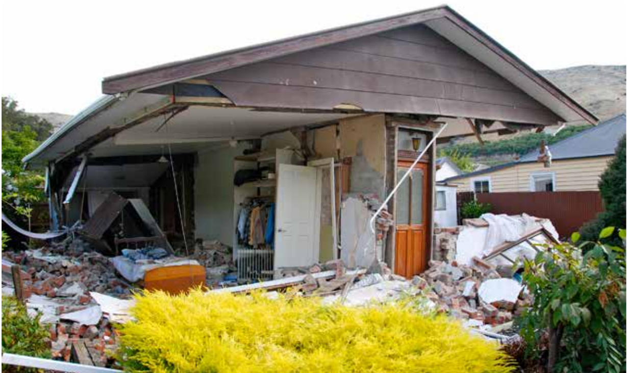
Damaged home in Heathcote Valley, where the February earthquake was centred.
