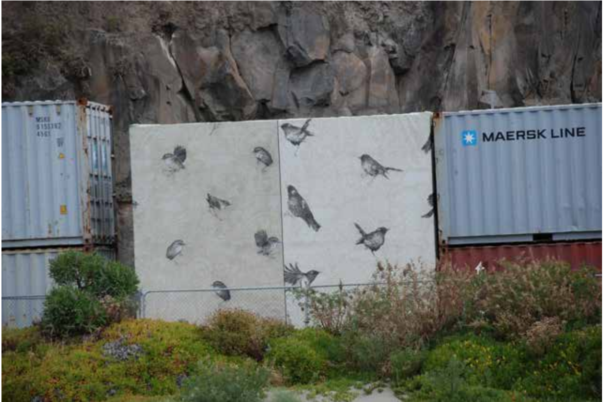
Container protecting the road from cliff collapse in Sumner.
