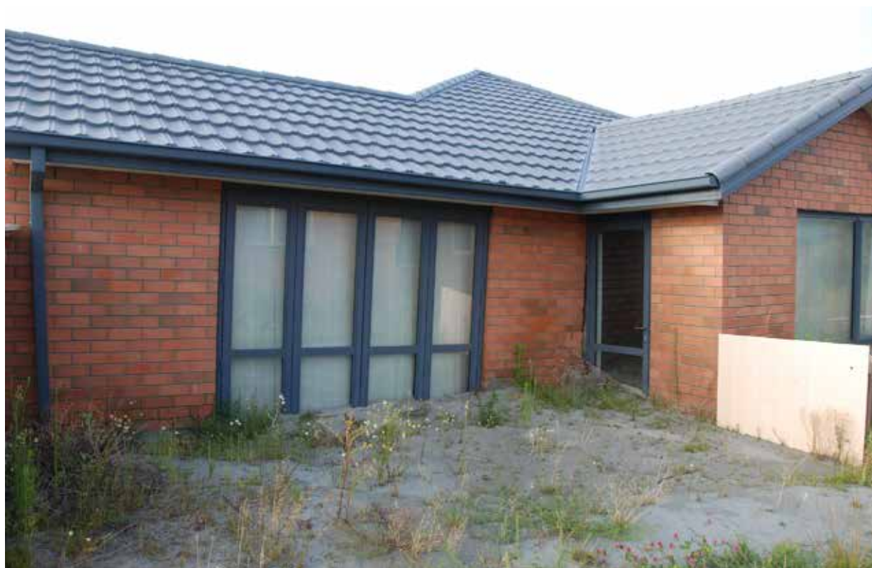
Home with liquefaction damage.
